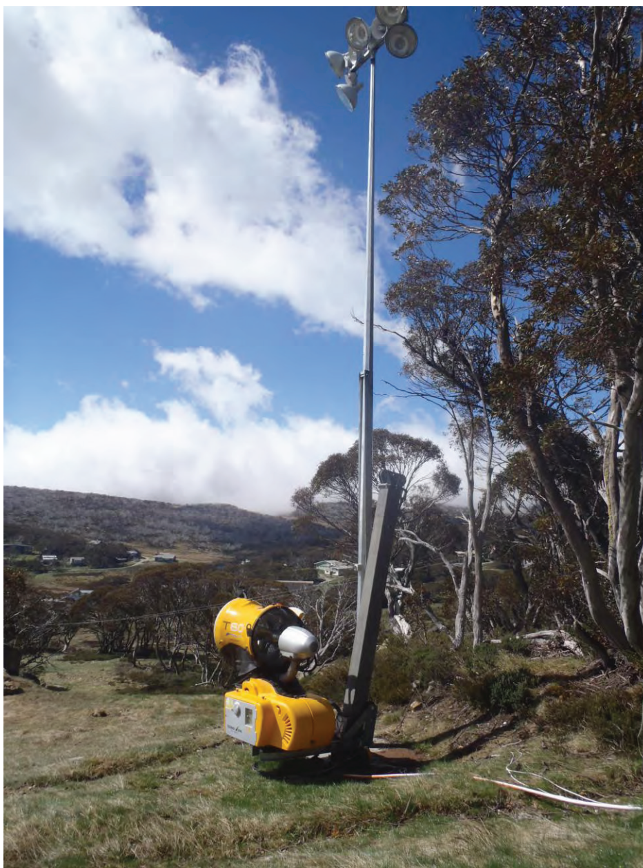
Figure 5: Existing fan gun and light pole (F1) to be removed and relocated
